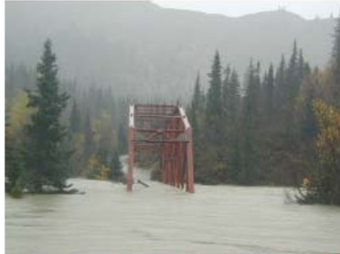
Photo 2: Iliamna Bridge 4 feet underwater, 2003 flooding.
