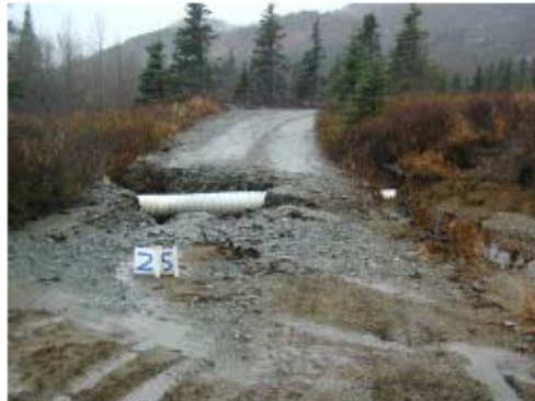
Photo 4: Williamsport Road washed out from 2003 Flooding.
