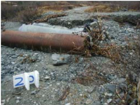
Photo 3: Williamsport Road washed out from 2003 Flooding.
