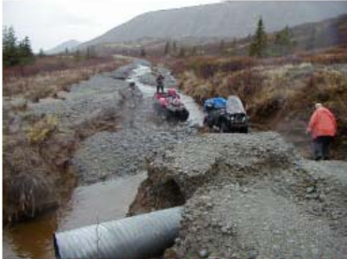
Photo 1: Williamsport Road washed out from 2003 Flooding.
